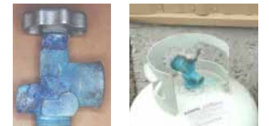
(Left) valve - (right) tank that has been exposed to Anhydrous Ammonia
