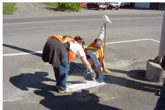
HBMI employee Sharri Venno and River Network's Angie Reed stenciling a storm drain in Houlton
